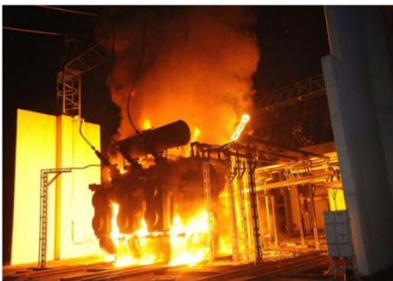
This Photo of an electrical station fire by Unknown Author is licensed under CC BY
